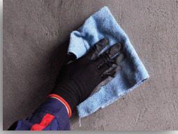
Ensure the surface to be treated is clean and free of contamination
